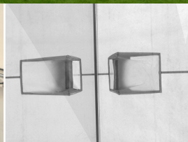
Venturi vents in the roof panels
