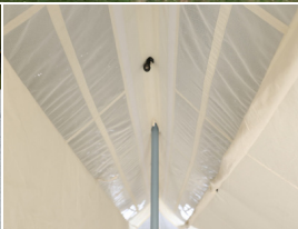
Ventilation strips along the ridge line.
